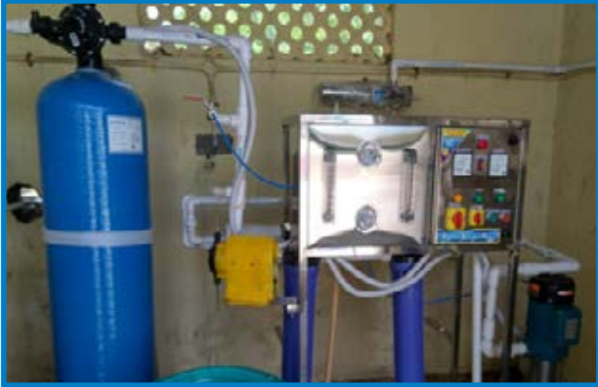
Photo 1 - RO Plant at OH, Karimnagar
