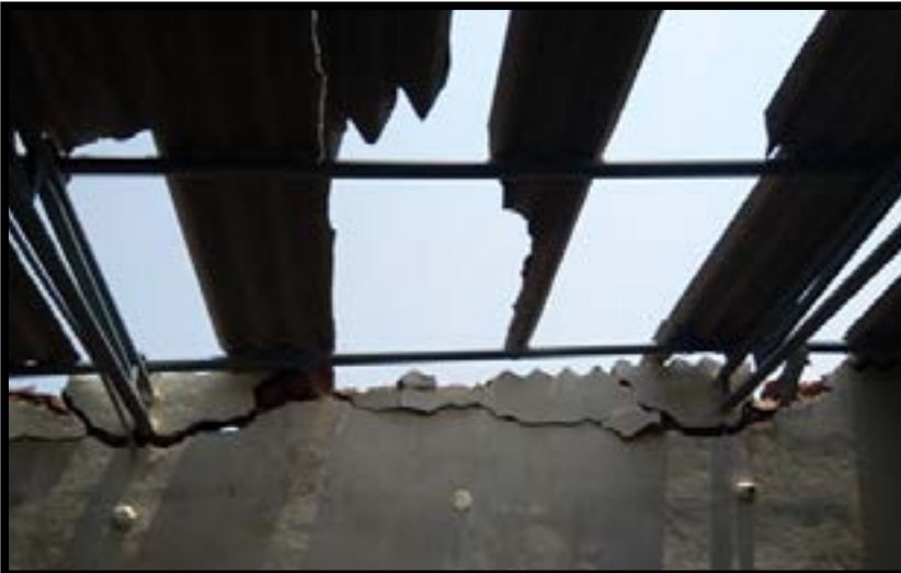
Photo 4 - Shattered roof of Vocational Training room at OH, Warangal
